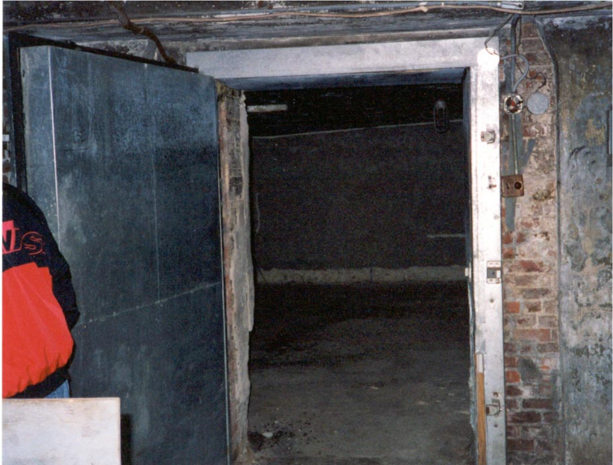
Photo 5. Cold-Storage Freezer Room
