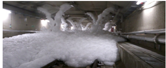
Figure 9 Testing the foam system in the Beveren tunnel in Antwerp.
