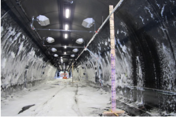
Figure 6 The If tunnel with the HotFoam® system installed. In the foreground can be seen one of the three depth gauges used to measure the foam depth, monitored by video cameras. Some foam is still left on the walls and floor of the tunnel after a test.
