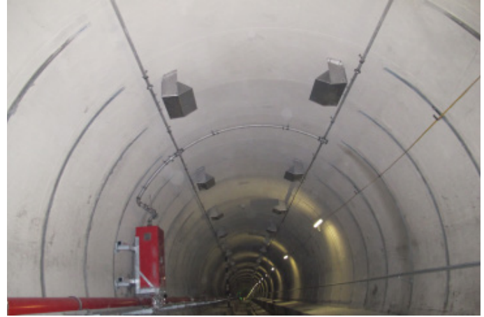
Figure 8 The foam system installed in the Boor tunnel in Antwerp.
