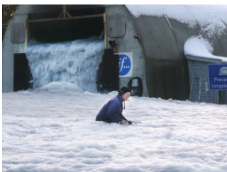
Foam firefighting system in rail tunnels ensures safe transport of goods to Europe.
