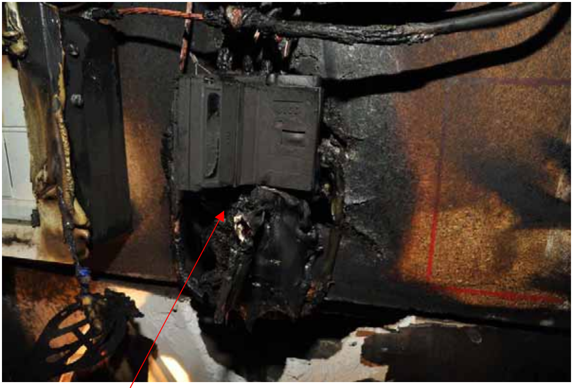
Damage to service head and cut out fuse
