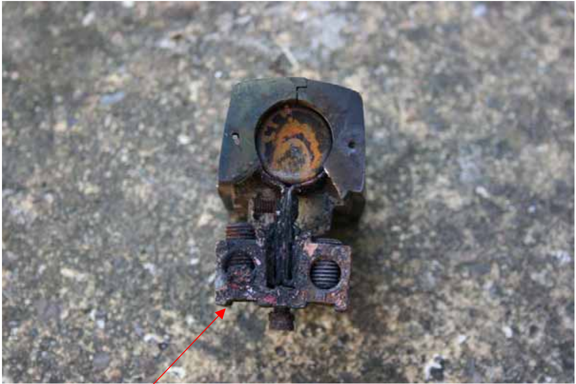
Oxidation to terminal caused by localised resistance heating
