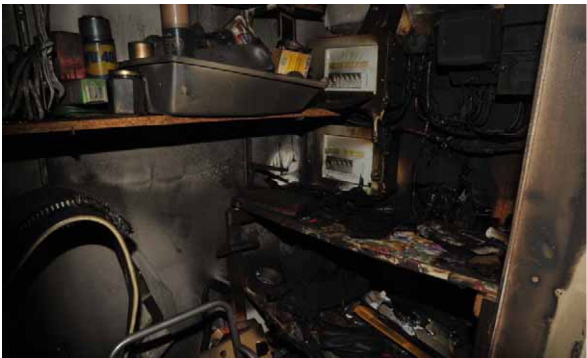
Cupboard housing electrical intake in hallway of flat
