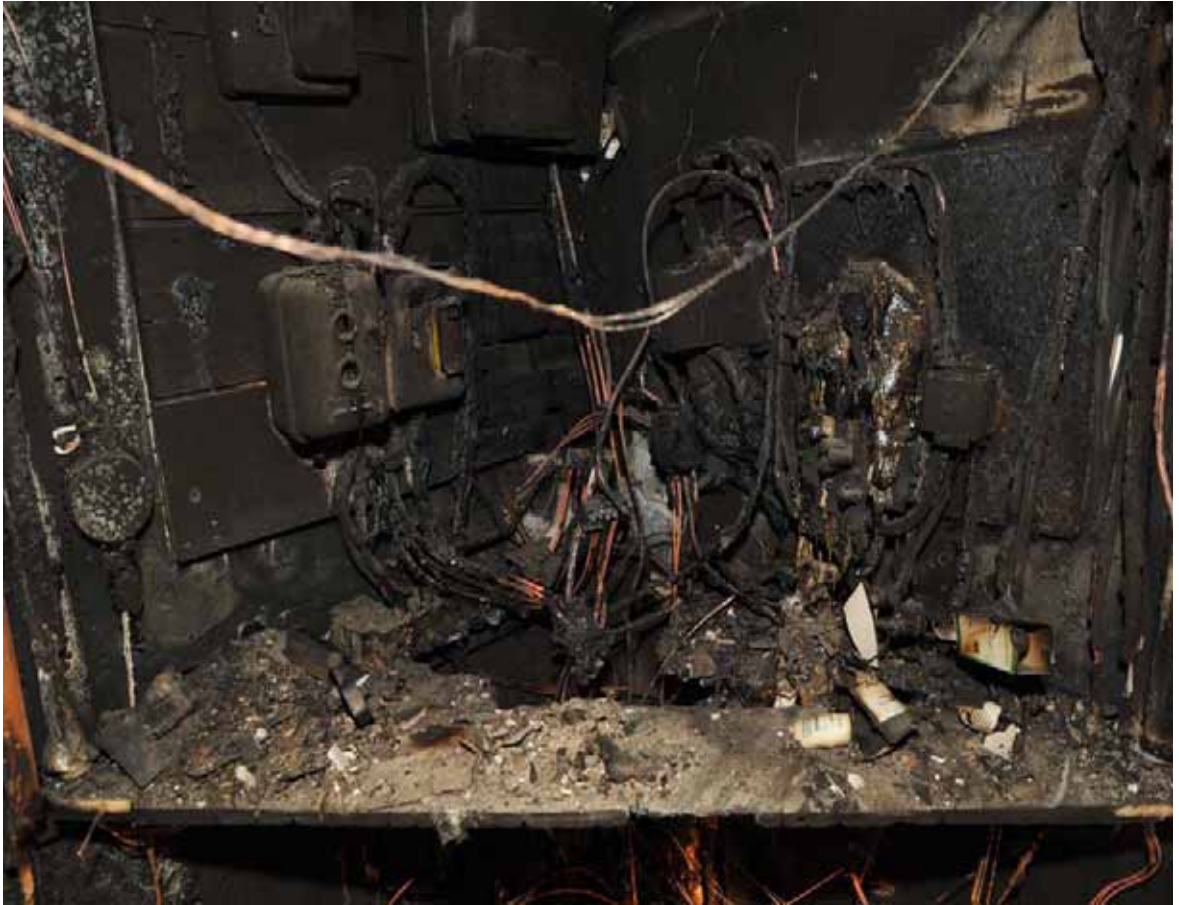
Widespread damage to electrical intake
