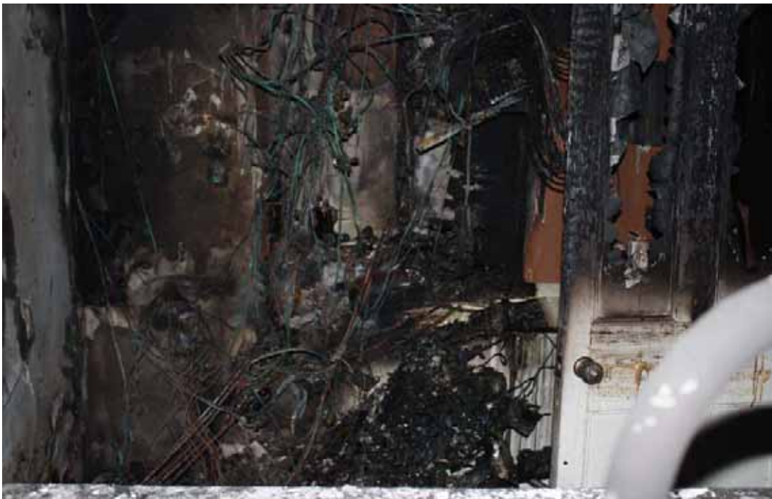
Fire originated in electrical distribution area and subsequently spread into roof
