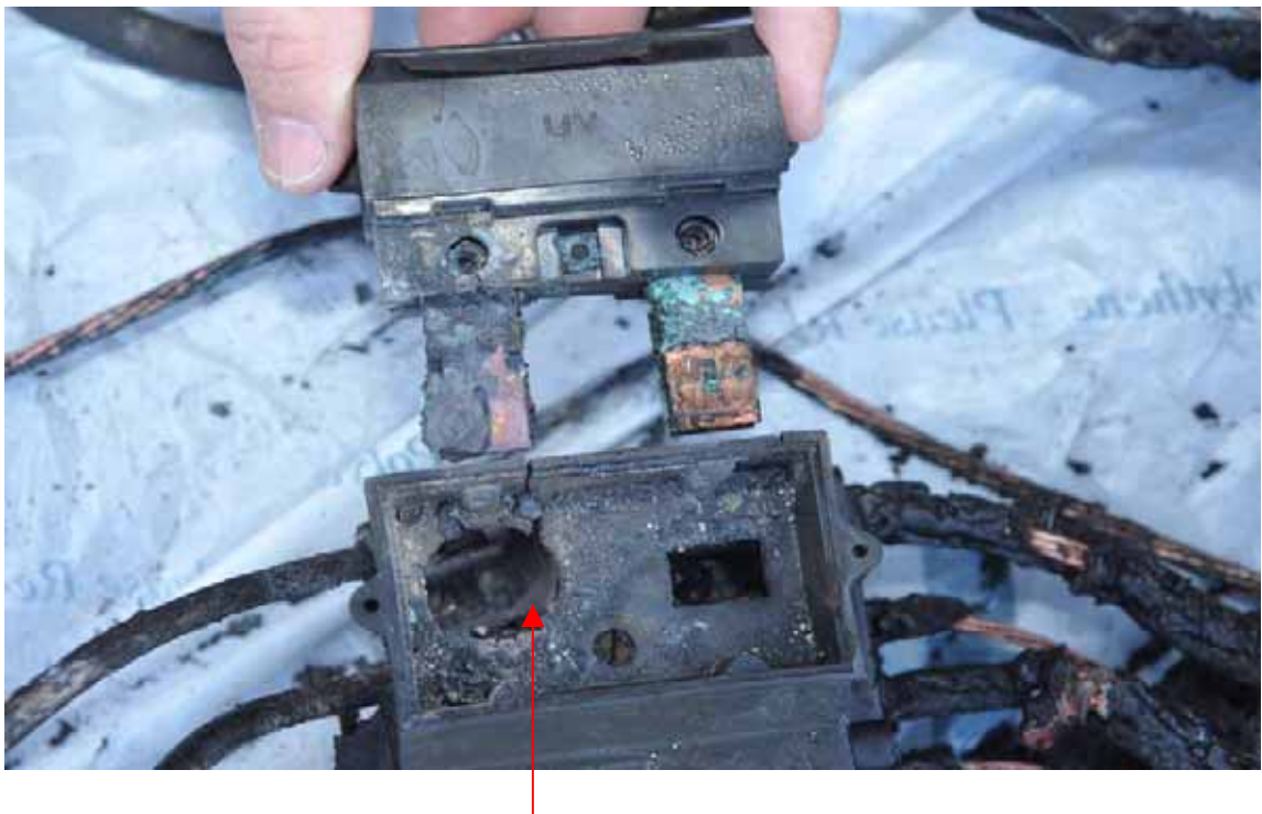
Cut out fuse showing heat damage to pin and holder
