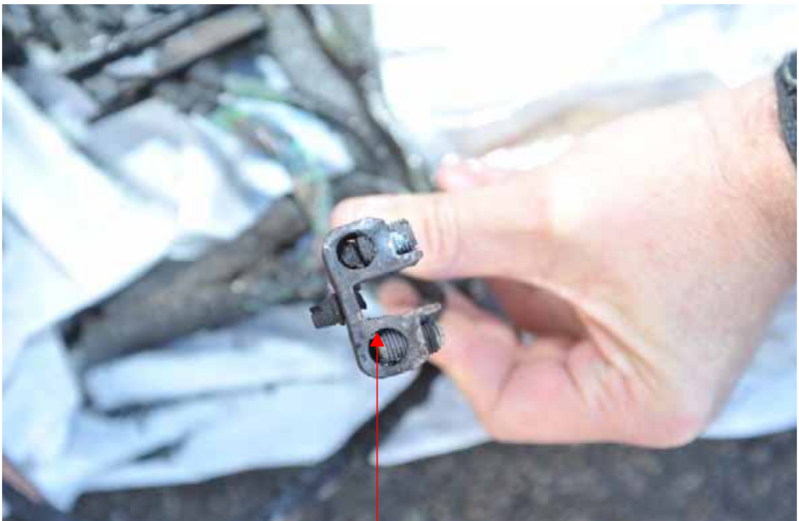
Terminal connection in cut out fuse showing screw not catching core
