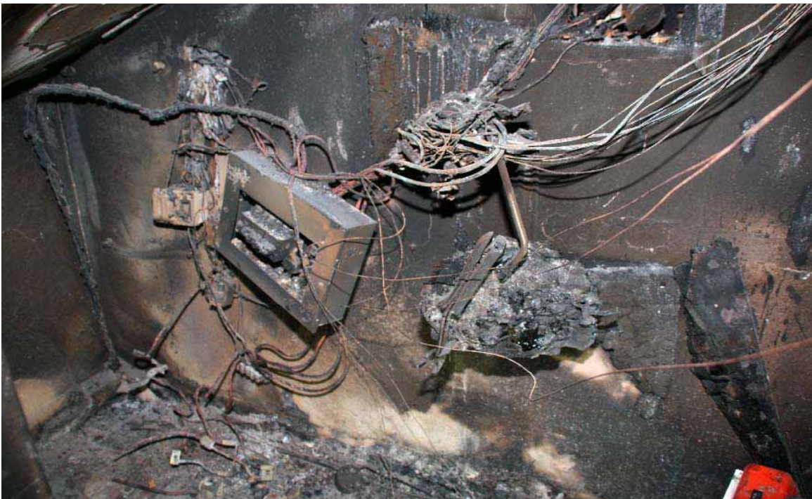
Seat of fire showing damage to electrical equipment in the under stairs cupboard
