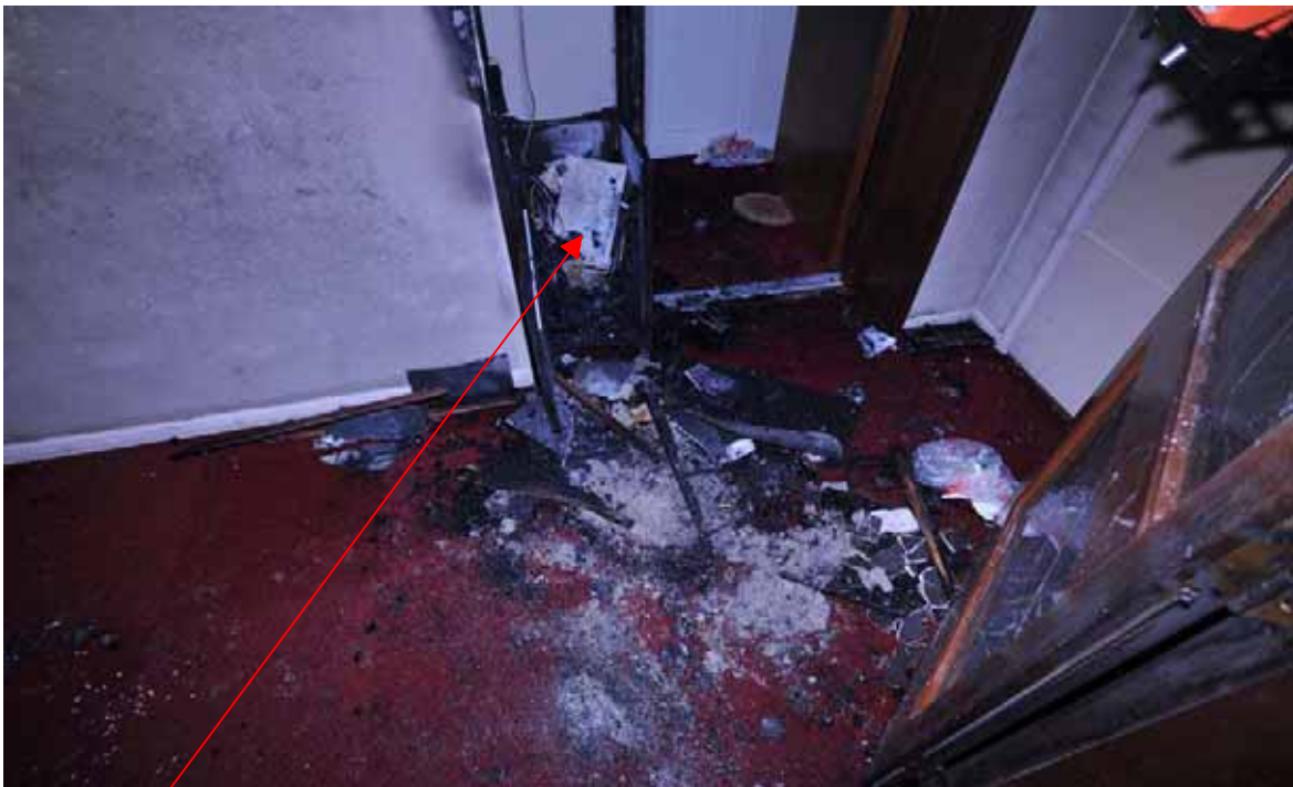
Damage to intake cupboard in common hallway on 5 th floor
