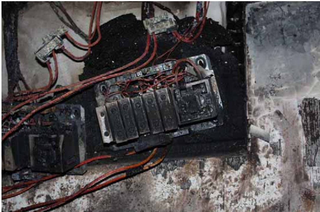
General damage to consumer unit
