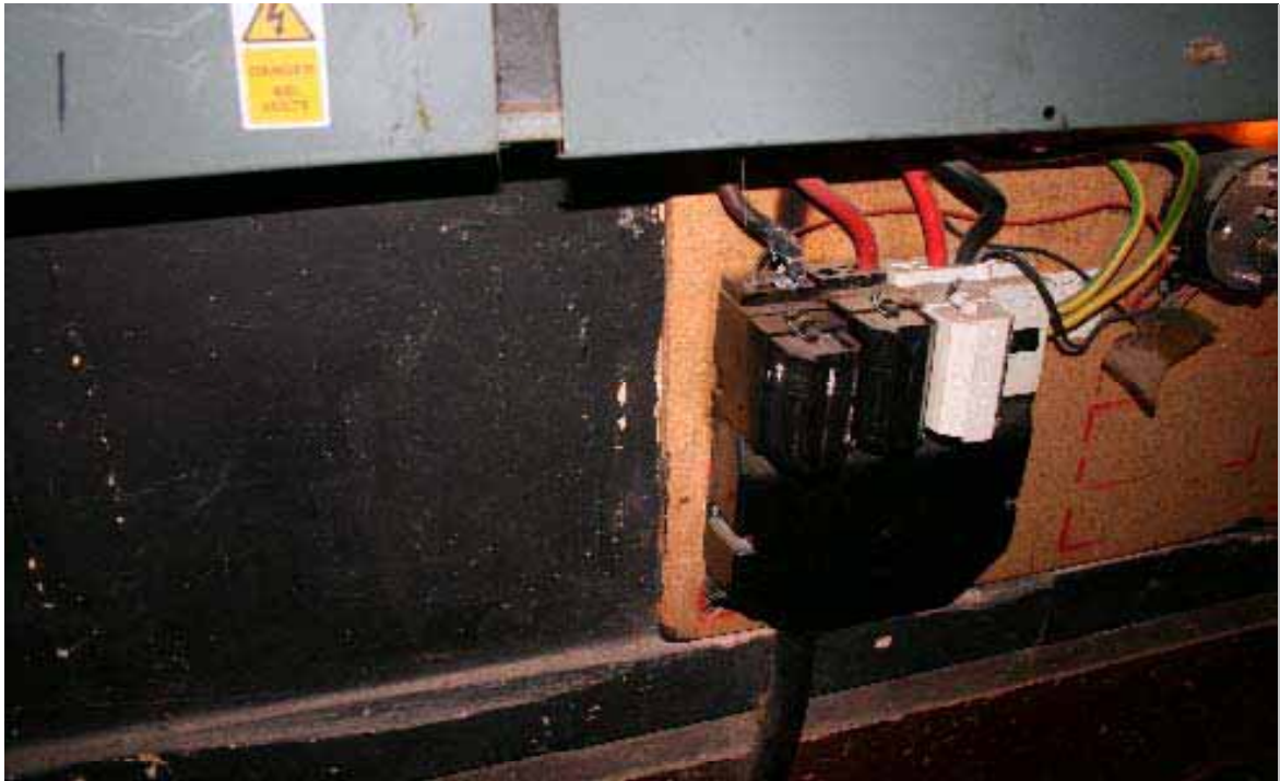
Cut out fuse showing overheated connection to cable
