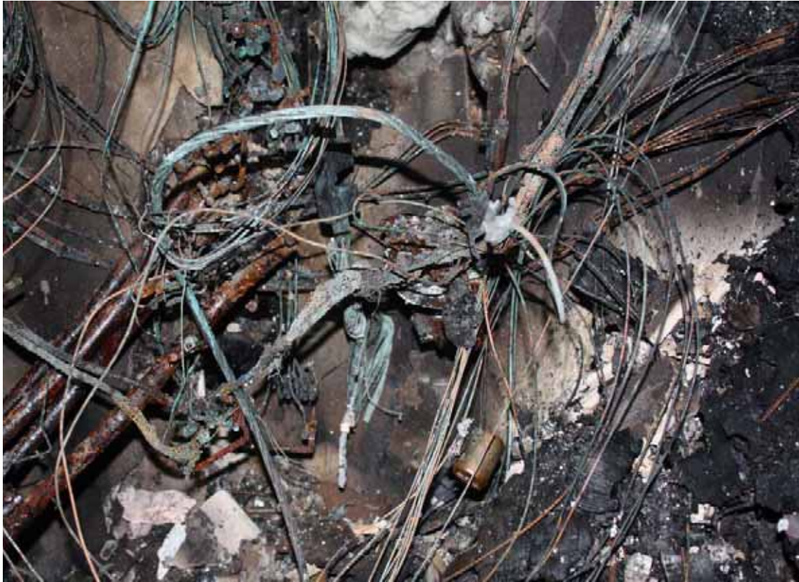
General and widespread damage to distribution area
