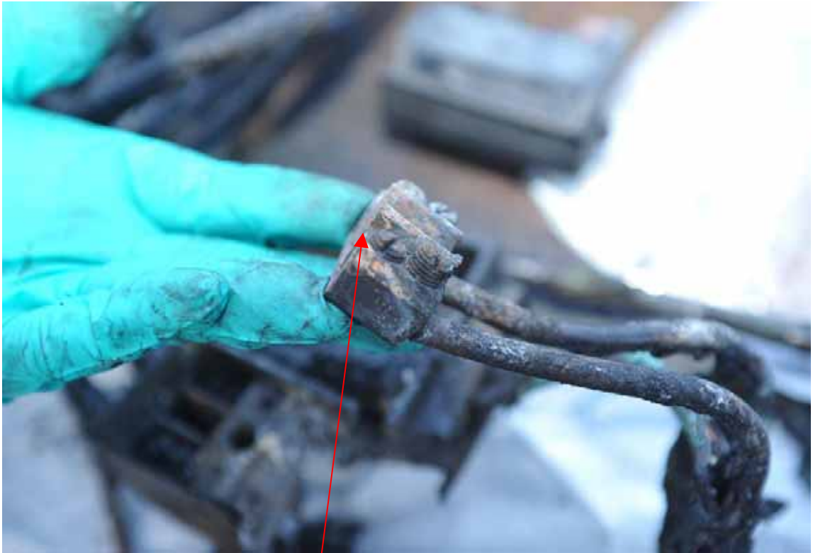
Terminal connection in cut out fuse showing screw not catching core
