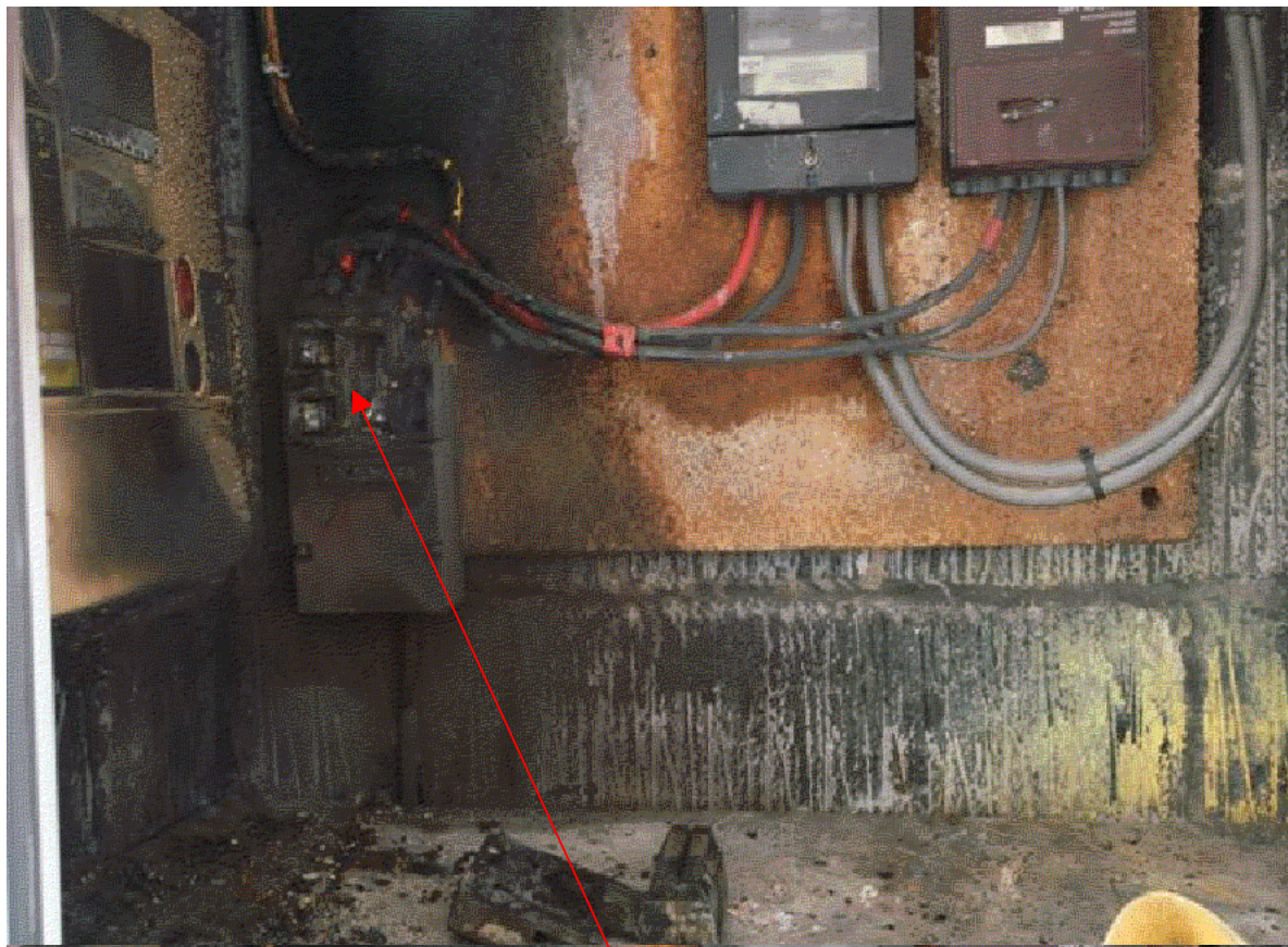
Photo taken by WSFRS showing damage caused by cut out fuse in a cupboard
