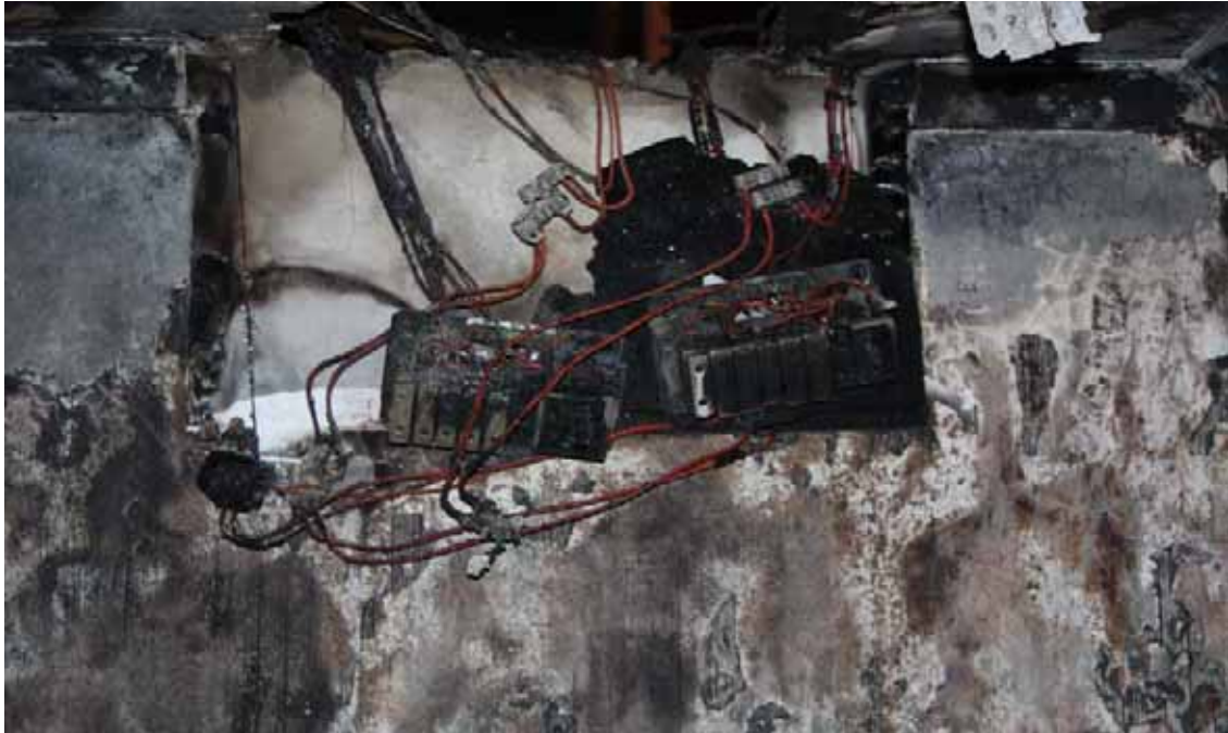
General damage to consumer unit
