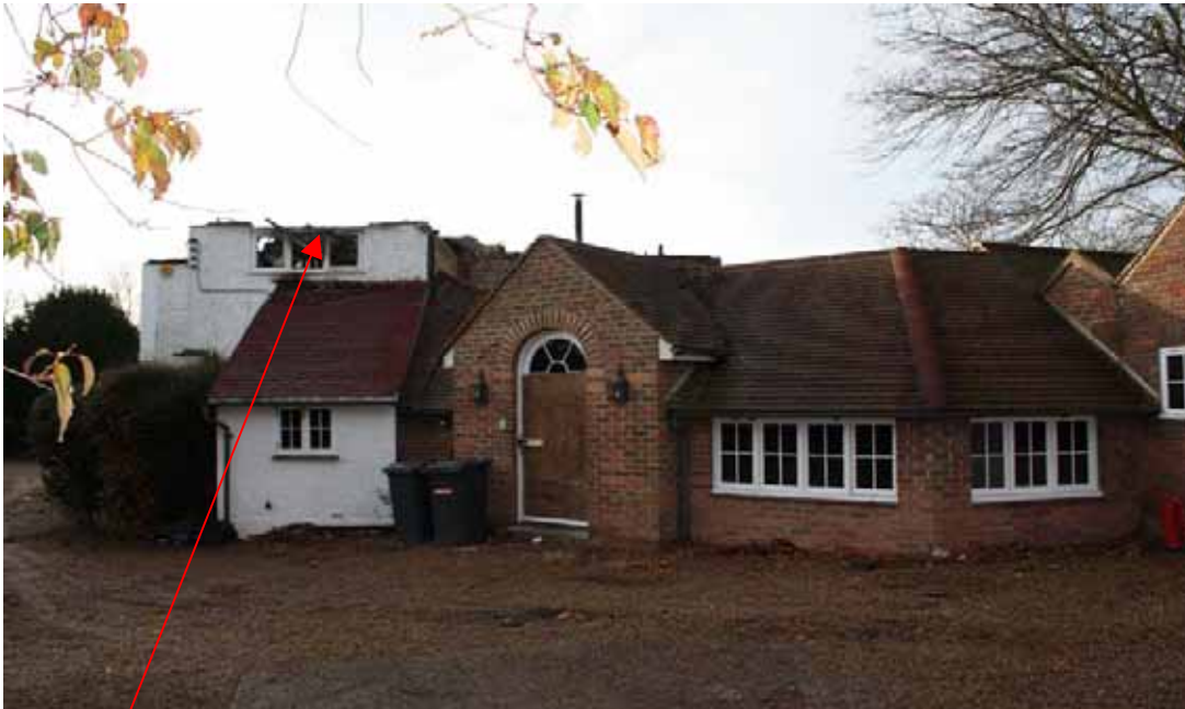
Roof destroyed and extensive internal damage through fire, heat and smoke spread
