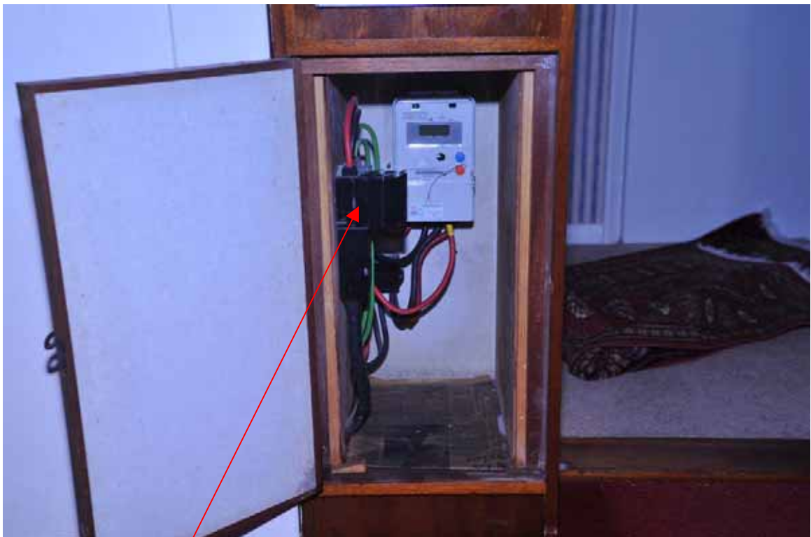
Example of cut out fuse in a similar electrical cupboard elsewhere in block
